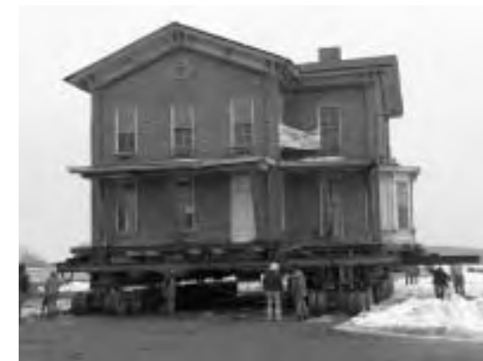
Relocating a 391-ton house is no small task, but well worth the effort to save the Smith House near Sun Prairie.
